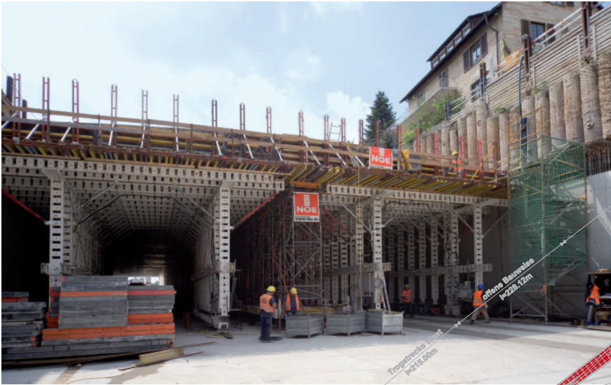
Formwork supported by loadbearing towers fills the gap in the area of the road alignment shift west
