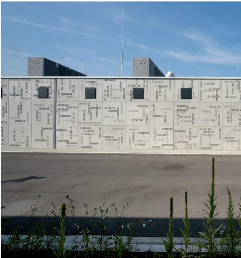
The raised and recessed binary numeric codes produce an interplay of shadow and emphasise the three-dimensional character of the concrete surface.
