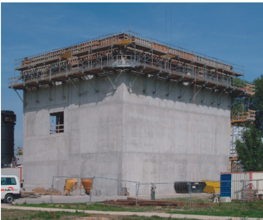
Scharnhäuser Park Combined Heat and Power Plant, Ostfildern-Scharnhäuser, Germany
